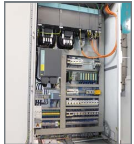
Schaltschrank Cabinet, in-house built
